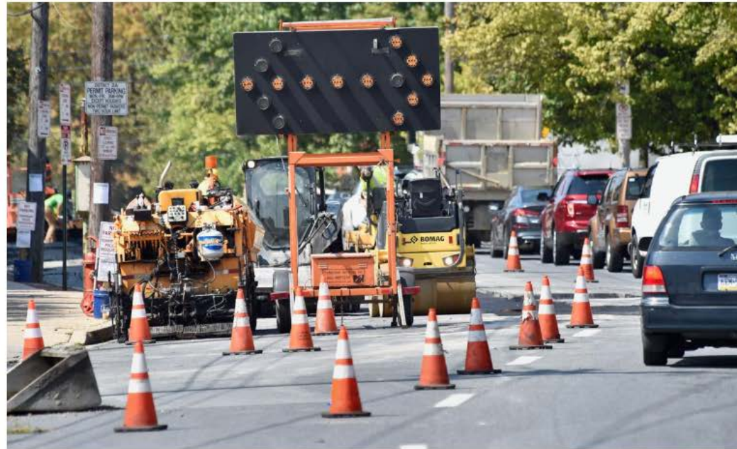
Construction workers from by B.F. Brown and Company, Inc. work to repave the 300 block of East Walnut Street in Lancaster city as motorists travel west after funneling into one lane on Monday, September 9, 2019.
